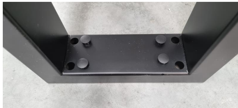
Base of steel frame where dyna bolts Are installed into the concrete floor. Also showing are the plastic covers
